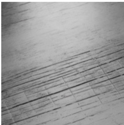
Weathered wood structure
